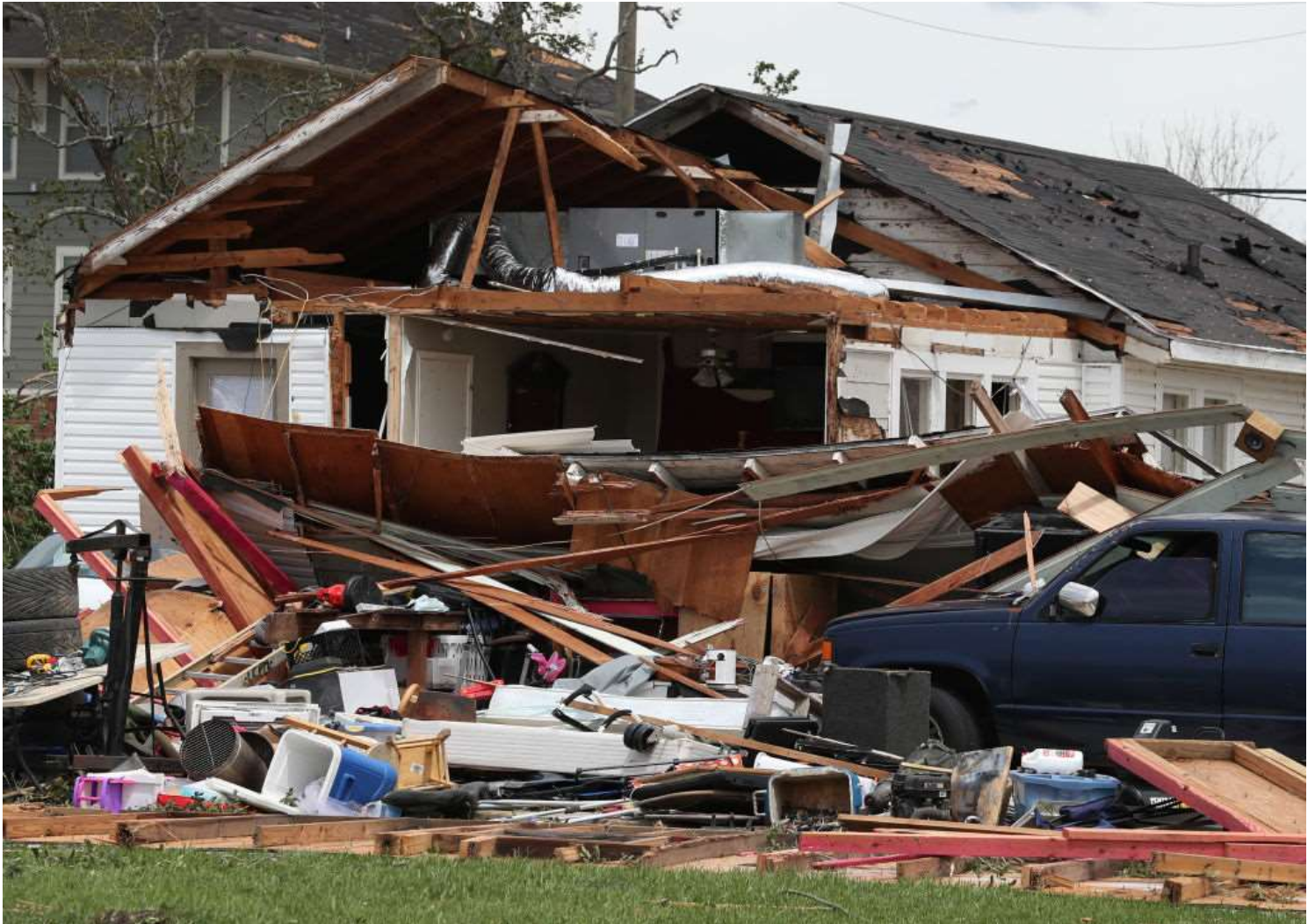
📷 A damaged home is seen after Hurricane Laura passed through the area on Aug. 27, 2020 in Lake Charles. The hurricane hit with powerful winds causing extensive damage to the city. (Photo by Joe Raedle/Getty Images)
